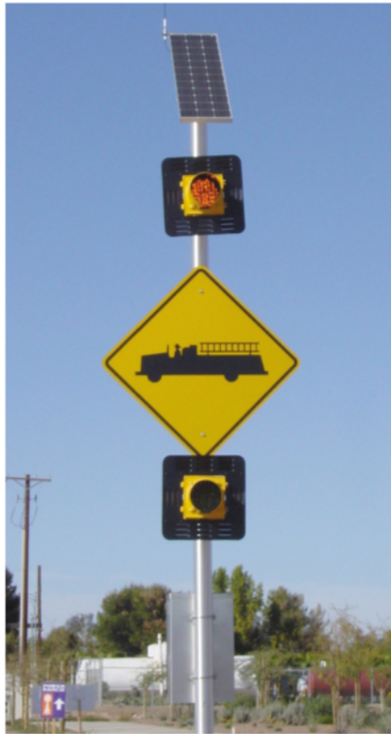
Typical Type I radio-activated fire station flasher.
