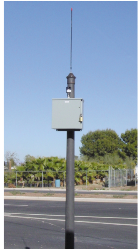
Optical sensor with radio transmitter at end of fire station driveway.
