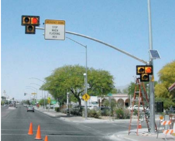
Figure 6, fire station exit signal system City of South Tucson.
