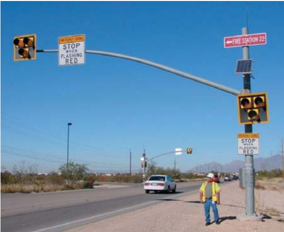
Figure 5, City of Tucson fire station exit signal with "Mickey Mouse" signal head.
