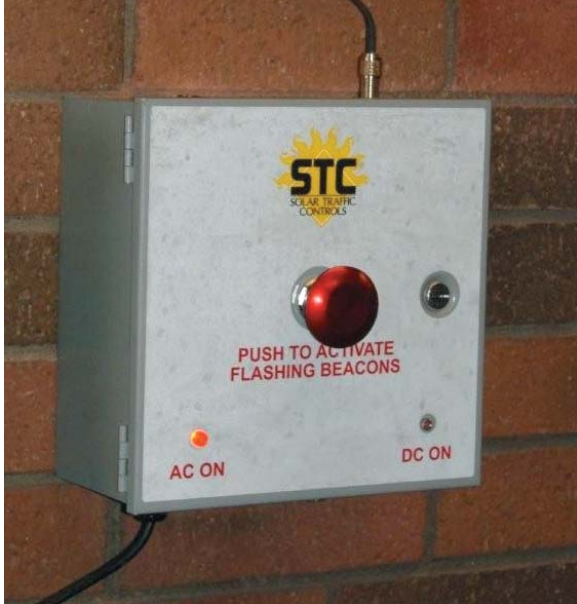
Figure 2, typical wall mount radio transmitter unit with roof-mounted antenna.
