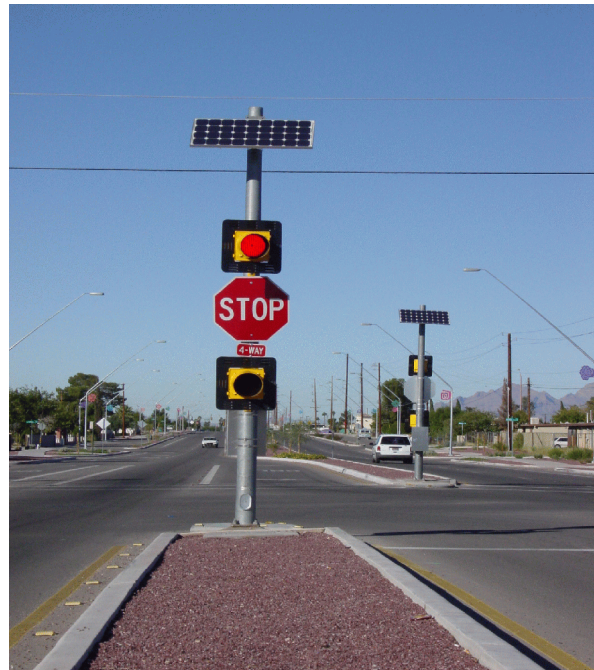
A properly working solar-powered flasher system begins with a clear definition of the desired result.
