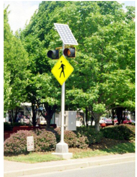
Dual 12-inch, flashing beacon system upstream from the crosswalk. Photo courtesy of Randy Dominick, Traffic Systems & Technology.
